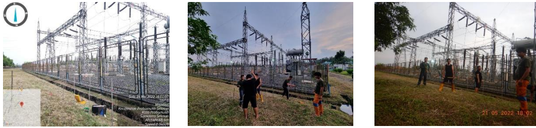
Figure 1. Location and Process of Testing and Measuring Grounding Resistance at Prabumulih Substation
