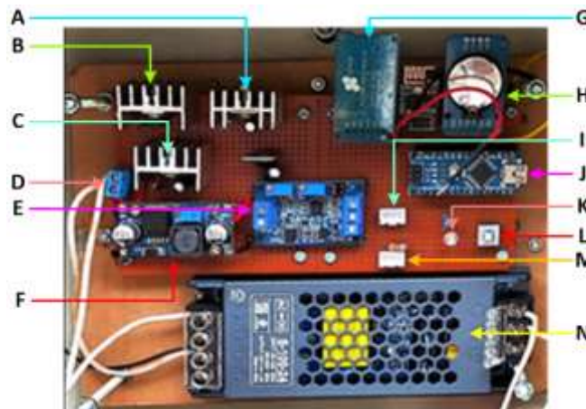
Figure 9. Data Logger on DC Panel Box
