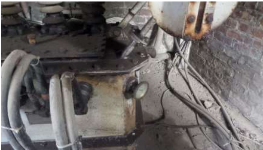
Figure 6. Snapshot taken during factory visit (Oil leaking in an old transformer)
