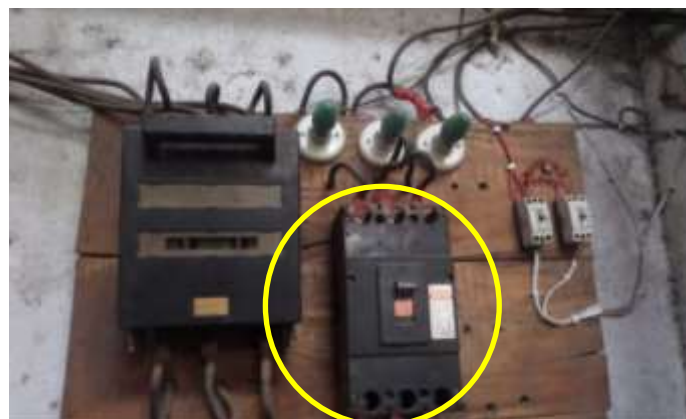
Figure 2. Snapshot taken during factory visit (Breaker capacity unknown due to altered label)
