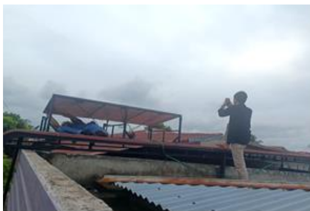
Figure 6. Rooftop solar panel 3 x 120 WP
